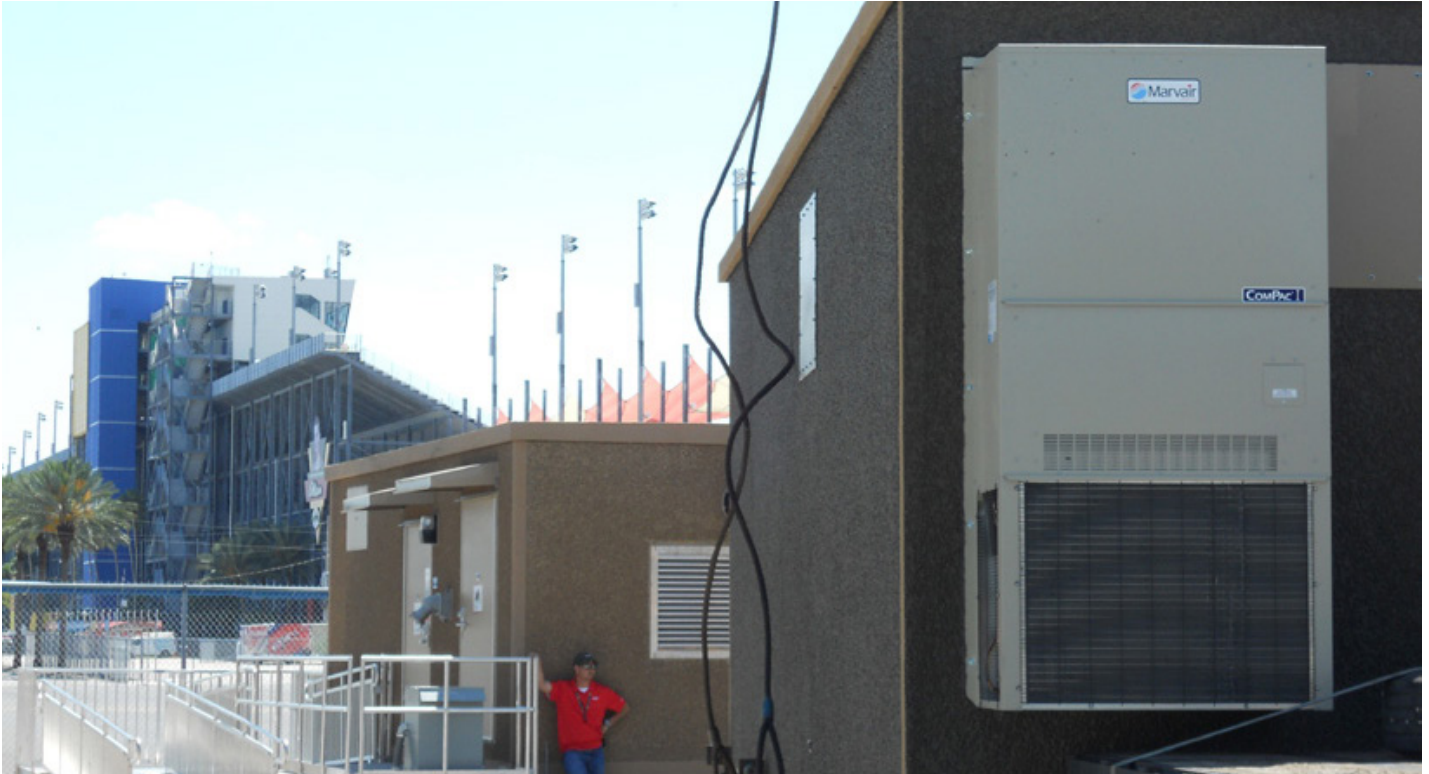
Turnkey - Distributed Antenna System (DAS) Network Buildings
