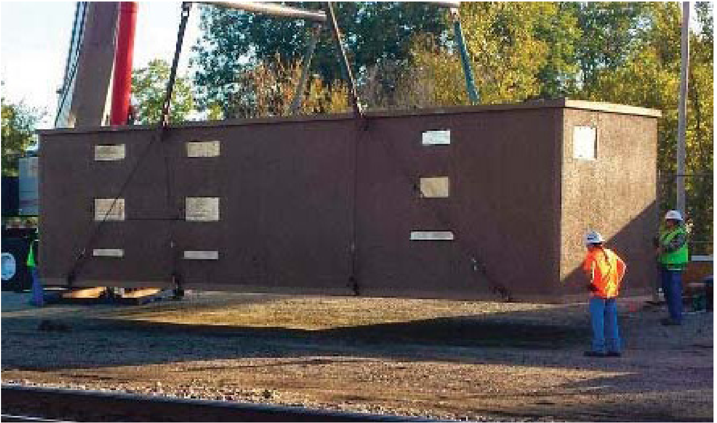
Communication Equipment Shelters and Fiber Optic Communication Lines within Existing Railroad Right-of-Ways
