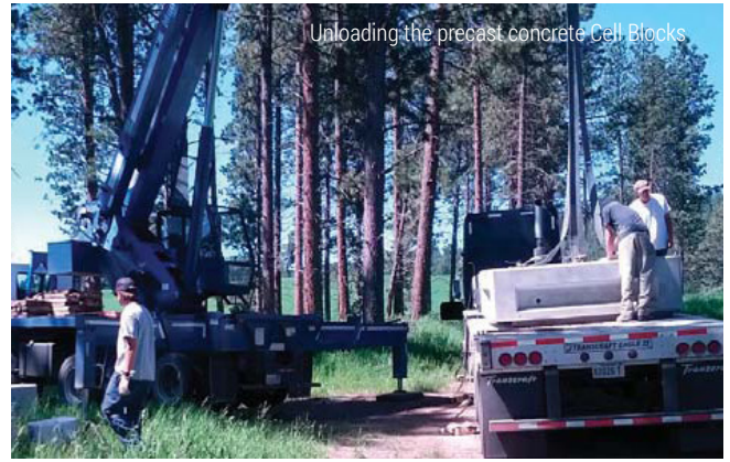
A 6-inch layer of granular material was placed on existing ground and compacted.
