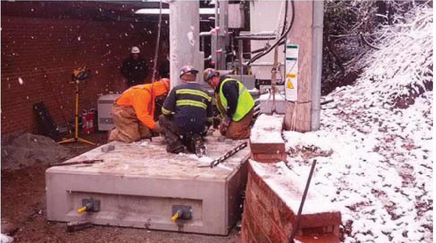
Cell Tower Foundation (Five Precast CELL BLOCK® Foundation) Placed and Post Tensioned in 90 minutes
