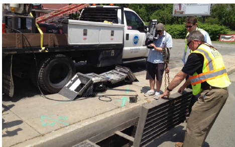
DPS crew installing FloGard +Plus catch basin insert filters along West Isabella Street
