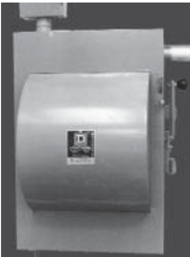
Manual Transfer Switch
