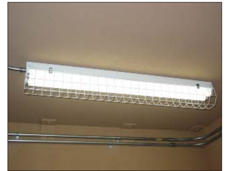
Interior Light with Wire Guards
