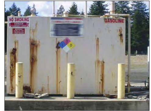
Rusted Steel Fuel Tank
