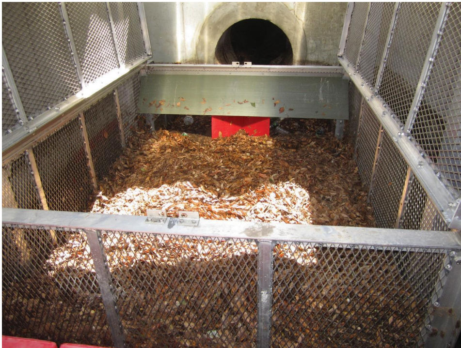
Nutrient Separating Baffle Box with trash / debris collected inside the screening system basket.
