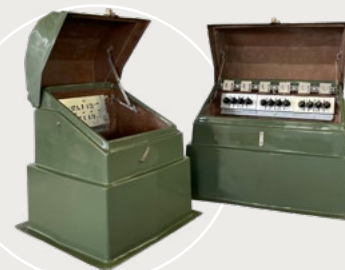
Sectionalizing Cabinets / Deferral Cabinets
