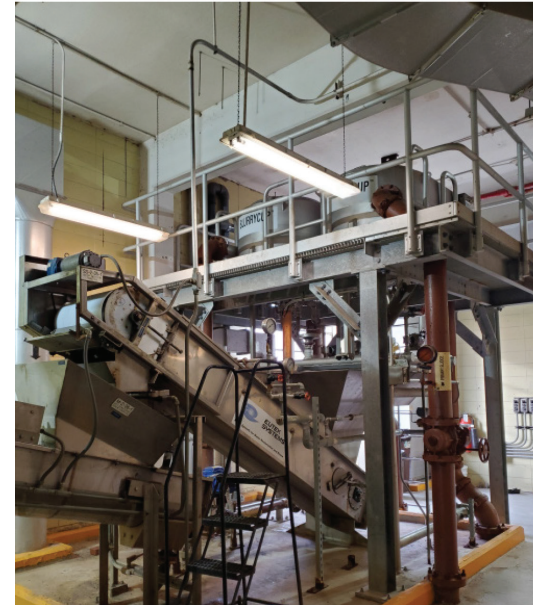
Clavey Road's Sludge Degritting SlurryCup / Grit Snail System in 2021
